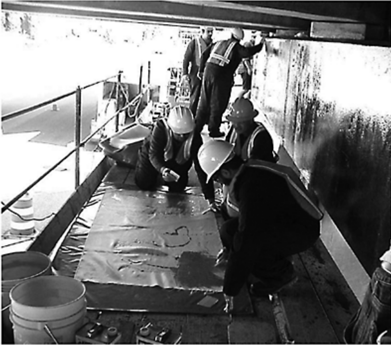
Figure 8.1 Retrofitting with composite material jackets: (a) hand lay-up of fiber-glass with epoxy by the authors; (b) machine winding of carbon fiber and epoxy (Source: XXsys Technologies, Inc., 1997).
