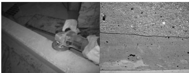
FIGURE 8.3 Grinding of concrete substrate surface (left) roughened vs. original concrete surface (right).
