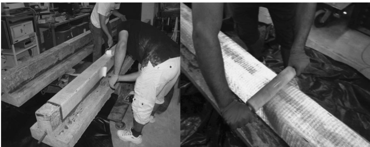
FIGURE 8.8 Applying resin to FRP with a paint roller (left) and clearing the air pockets with a wooden roller (right).
